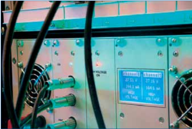
Close-up view of a dual channel high voltage Booster
